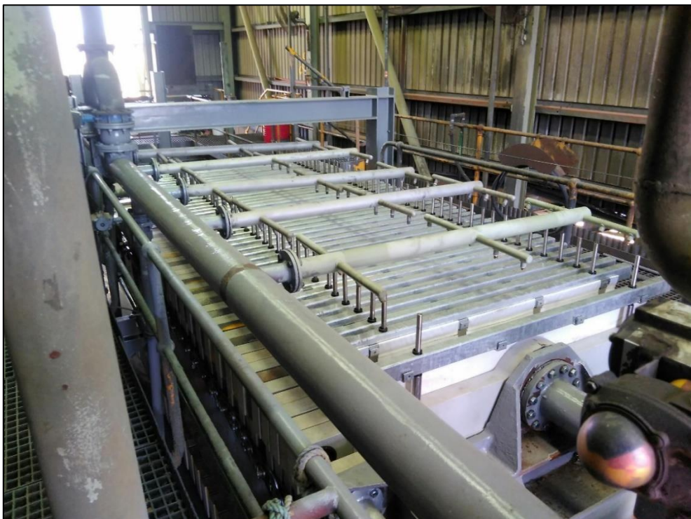
Photo 5 - Refurbished concentrate filter press
