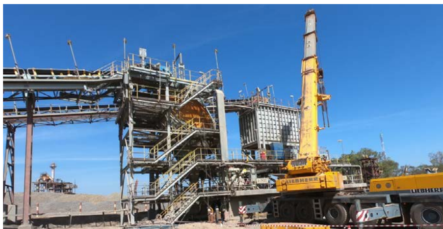
Figure 5: Syama Sulphide crushing circuit - new HP5 crusher installation
