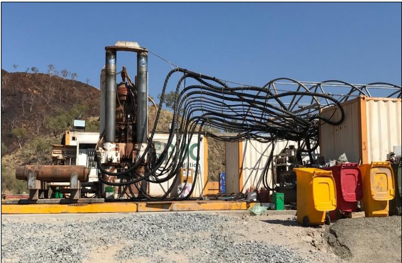
Figure 2: Raisebore drilling the pilot hole for the Savannah North Ventilation Intake – September 2018
