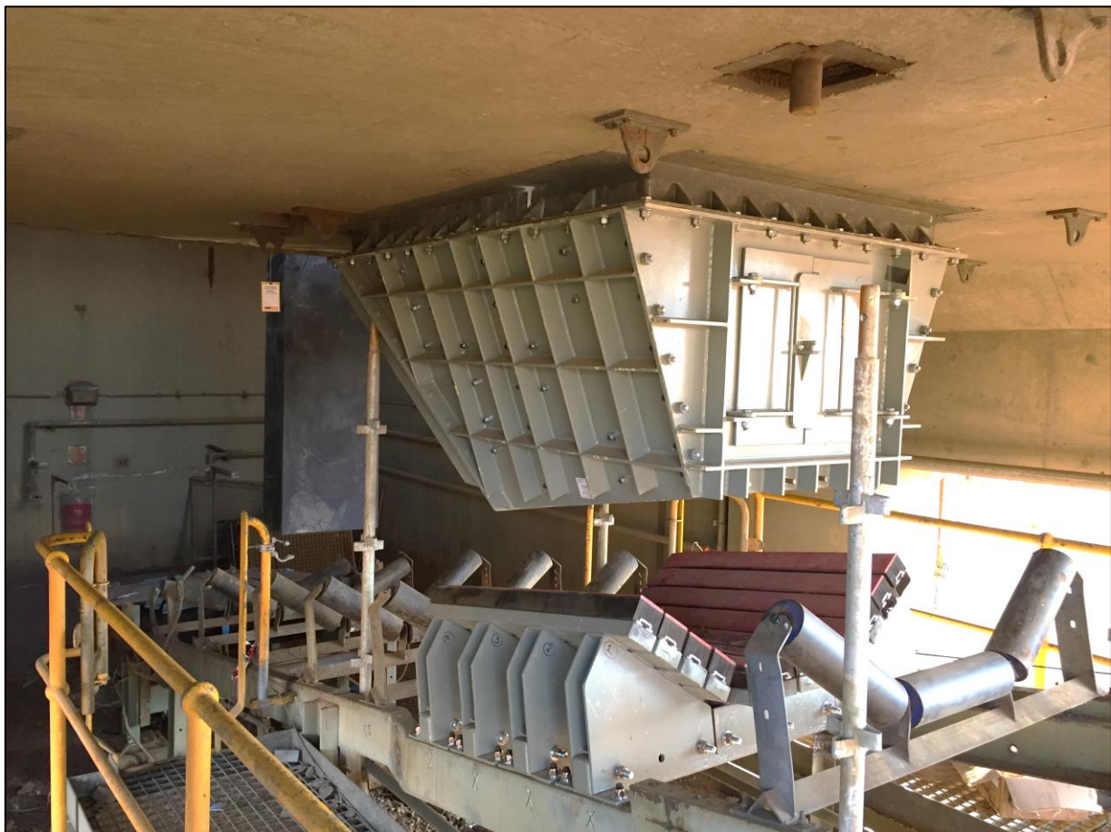
Figure 1: New feed chute and impact beds installed under the Ore Crusher – October 2018
