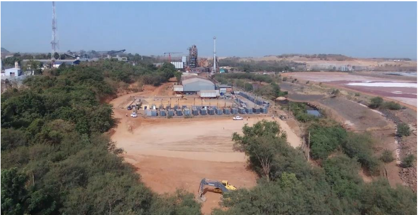
Figure 5: Earthworks underway at the new Syama Solar-Hybrid Power Station and HFO fuel Farm
