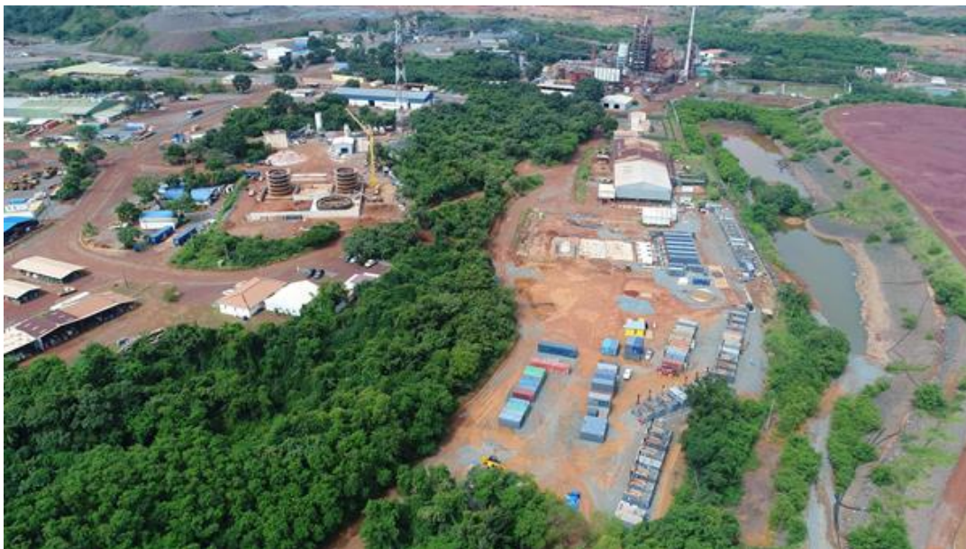
Figure 5: Earthworks continues at the new Syama Solar-Hybrid Power Station and HFO fuel Farm
