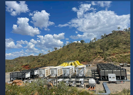
6MW Chiller Plant
